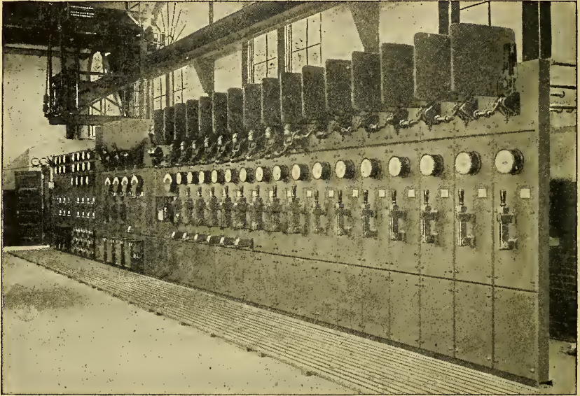
FIG. 320.—This front view of a switchboard for a railway power plant shows the feeder panels, with their switches and circuit-breakers in the foreground, the station metering panel in the center of the board and the generator panels in the background.
